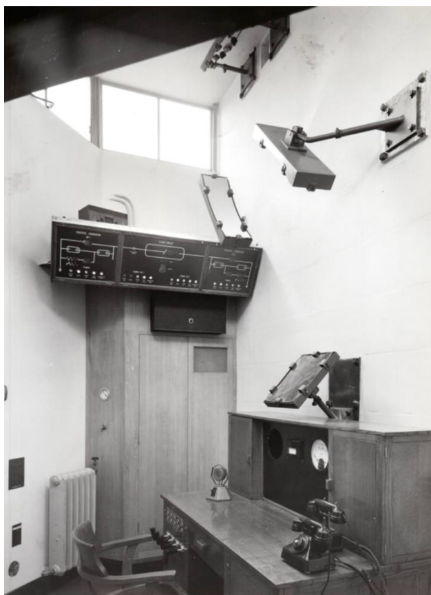
Fig 27. Photograph of control room showing dose rate meter; microphone for communication with patient; simple circuit with lights to show any faults; a periscope system of mirrors to view the patient on the other side of the barrier. (Barts Health NHS Trust Archives)
